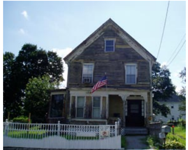
Owners of dilapidated structures should be informed about possible building code violations.
